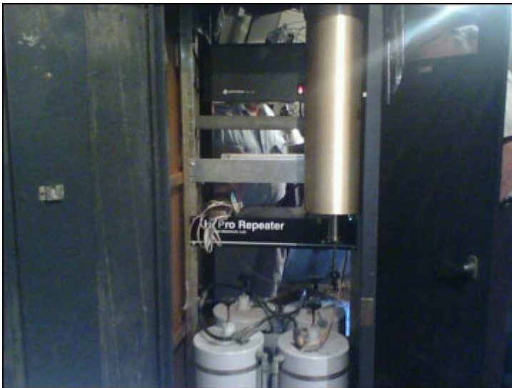
This is the front side of the Repeater. From top to bottom, one will see the power supply, controller, repeater, and finally the duplexer. The can at the top right is an extra filter used to help with some intermode problems we had with the old repeater.
